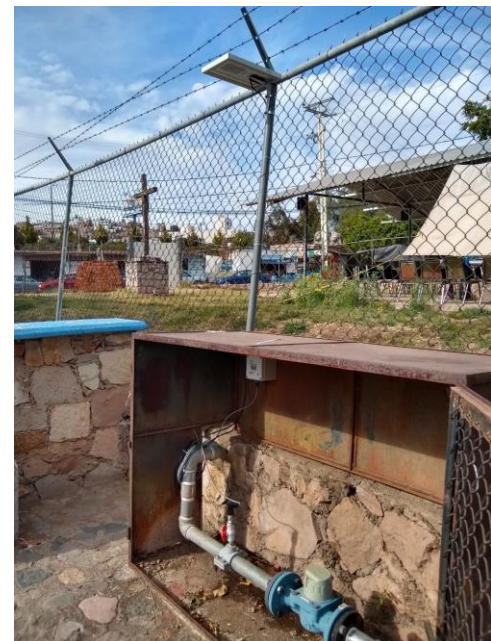
Fig. 4. Second IoT station.
